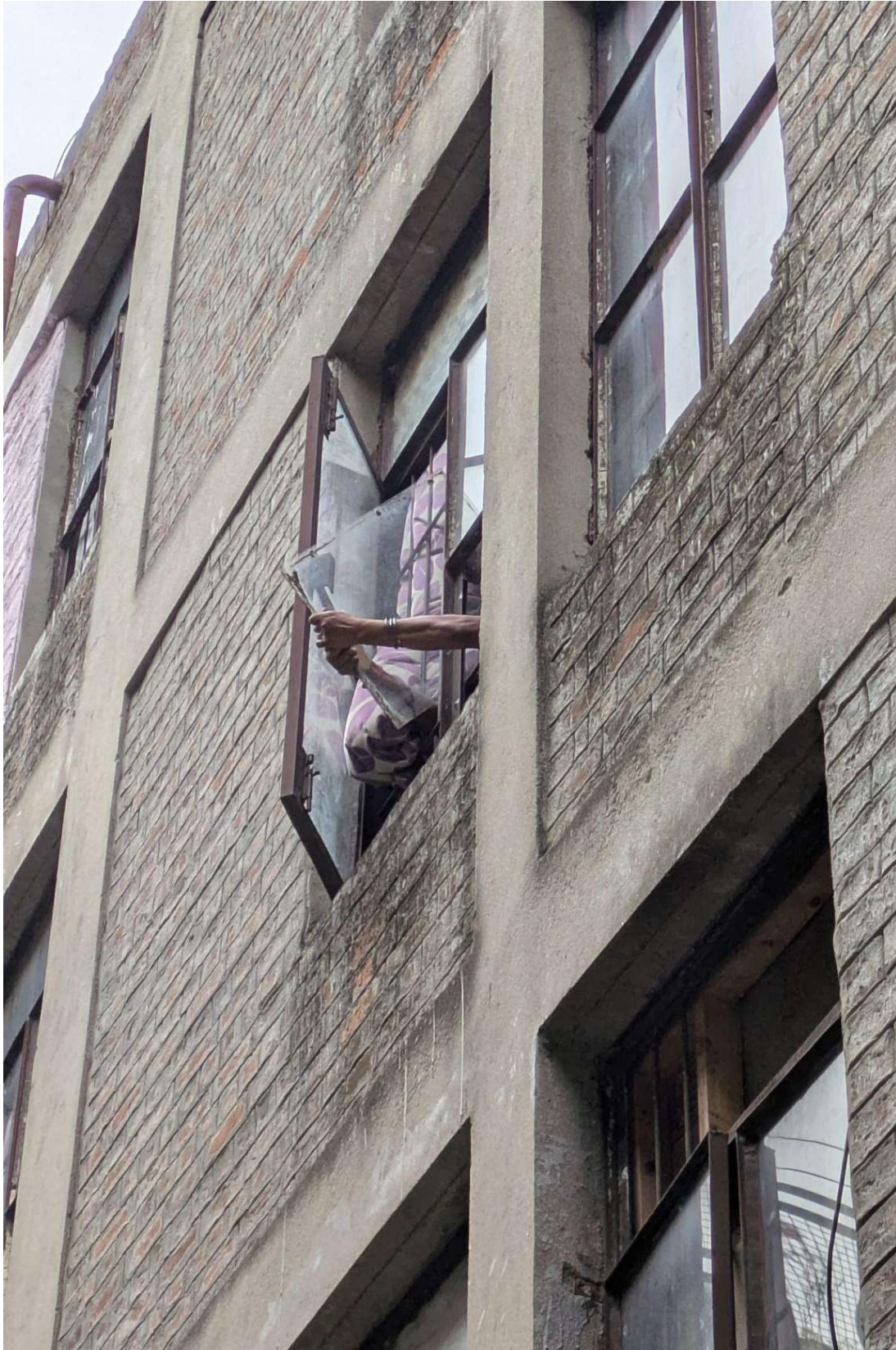
Figure 21: A resident in ARHC housing taking out the glass pane during heavy winds, fearing it might fall
