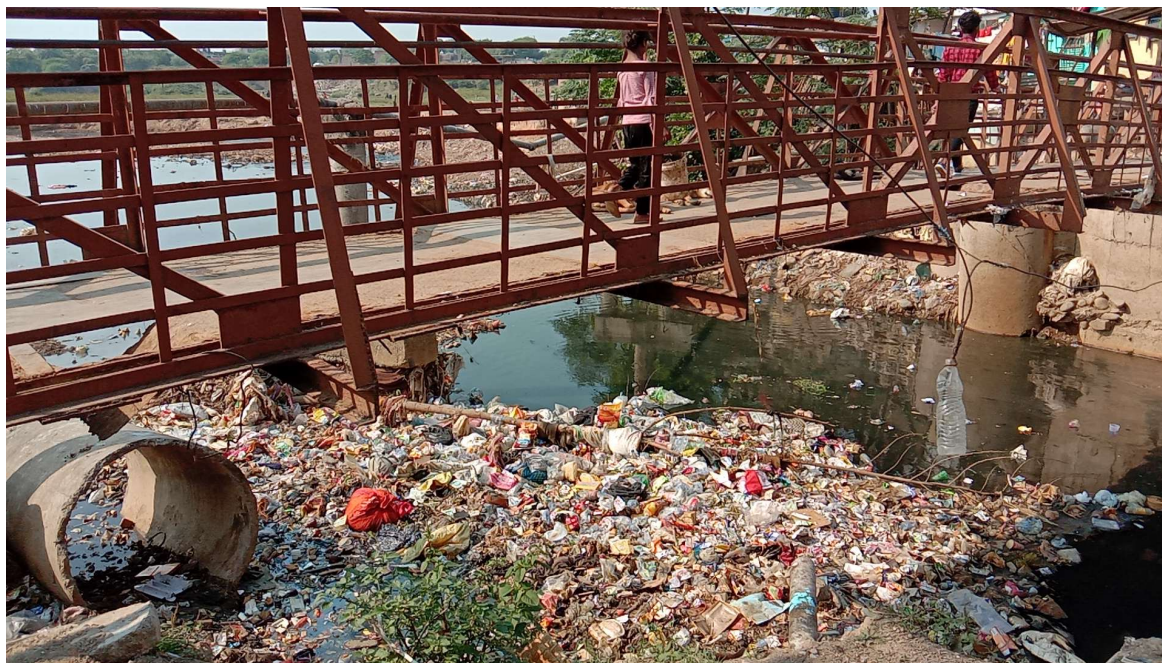
Figure 14: Drain filled with waste in Faidan Nizampur, a peripheral urban village in Chandigarh
